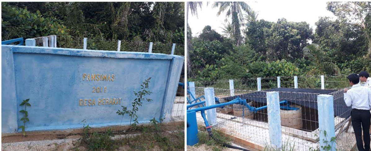
Figure 4. Pamsimas Infrastructure in Berakit Village.
